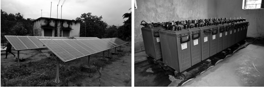
Figure 3.2 Photographs of a mini-grid at the field-site. Notice the solar panels on the ground and a battery-bank inside a control-room.
