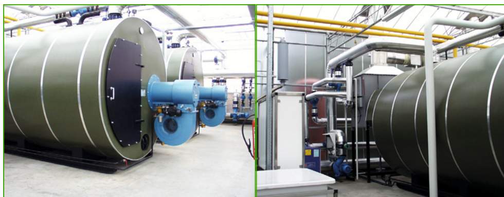
Figure 8.8. A twin central hot water boiler with (internal) flue gas condenser (left). Insulated distributor and collector pipes and flue gas unit (right). (photos: Bert van 't Ooster)
