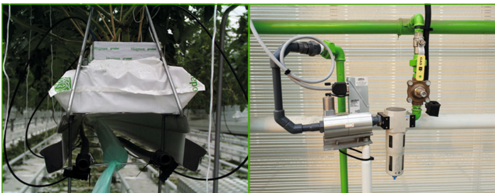
Figure 11.4. The distribution system for CO 2 in the greenhouse. Left: the polyethylene ducts for distribution of flue gases (green), placed below a crop gutter. The two irrigation lines (black) can also be seen, and the 'spaghetti' for the drippers. Right: mass flow controller for pure CO 2 . (photos: Frank Kempkes, Greenhouse Horticulture, Wageningen University & Research)
