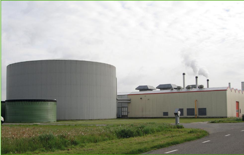
Figure 11.2. Heat storage tank, which is a well-insulated water tank (the largest cylinder in the picture), towering over the technical space housing the co-generator of a large greenhouse complex in the Netherlands (photo: Paolo Battistel, Ceres s.r.l.).
