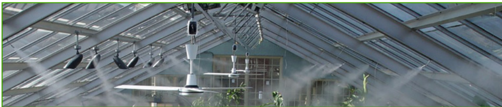
Figure 4.11. Example of a fog system actively spraying fine droplets in a greenhouse.
