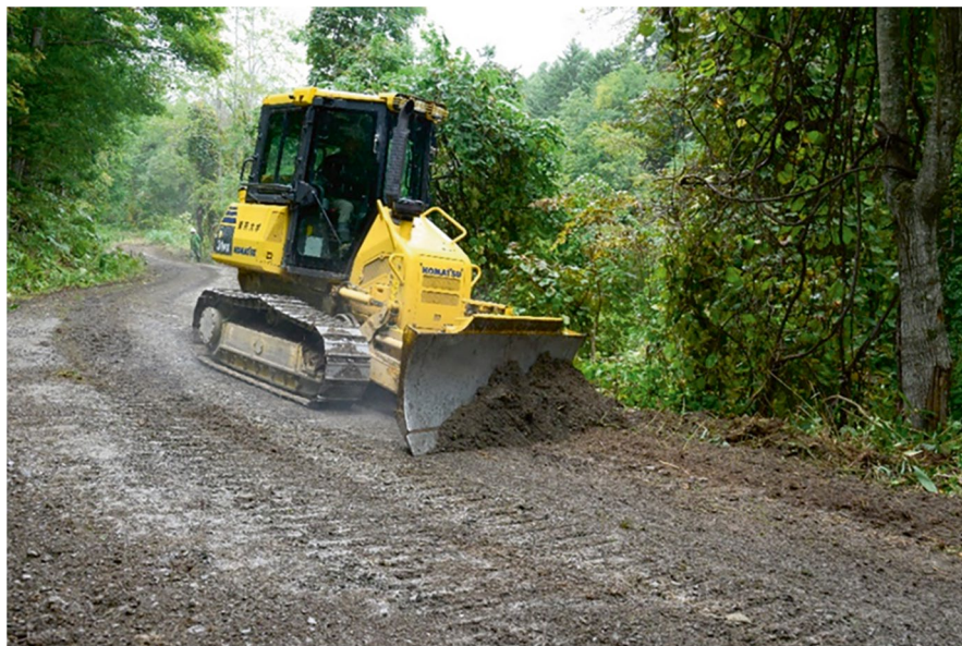
Fig. 9.9 Road surface maintenance performed by a bulldozer. (Photo by the UTHF, licensed under CC BY-NC-ND 4.0)
