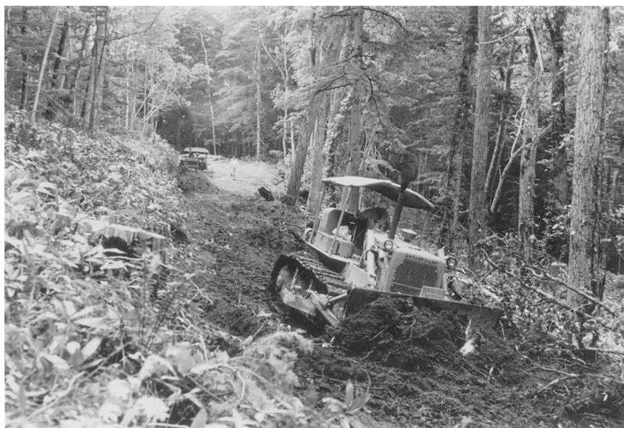
Fig. 9.7 Forest road construction using two bulldozers in 1968. Front: CAT D6c; Rear: Komatsu D50A, Compartment 41. (Photo by the UTHF, licensed under CC BY-NC-ND 4.0)
