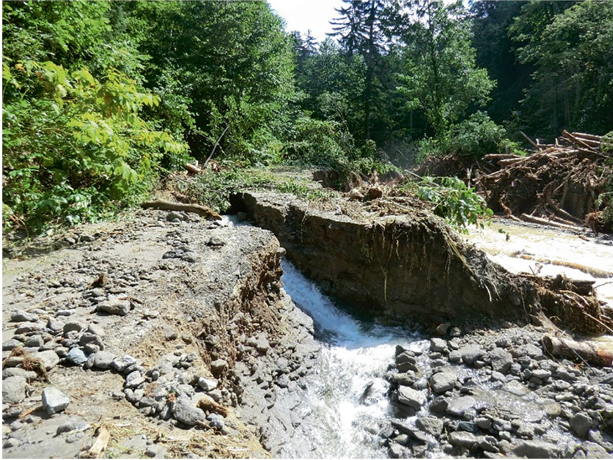
Fig. 9.10 Forest road disrupted by successive typhoons in August 2016 (Compartment 92). (Photo by the UTHF, licensed under CC BY-NC-ND 4.0)
