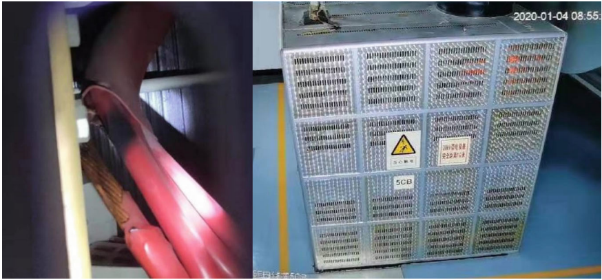
Fig. 6.7 Transformer discharge fault images
