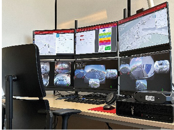
Fig. 2 Operating Control Centre (OCC) at Les Mureaux. Source Transdev
