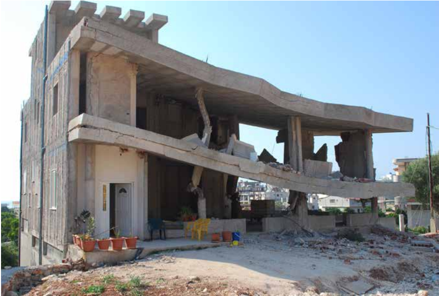
FIGURE 2.3. Collapsed house, still inhabited, Ksamil, 2010. © Francesco Vietti
