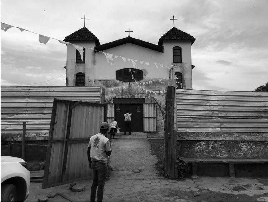
FIGURE 9.1 Catholic church still damaged almost three years after the Mariana dam break, in Brazil Source: photo by Victor Marchezini (1 October 2018)
