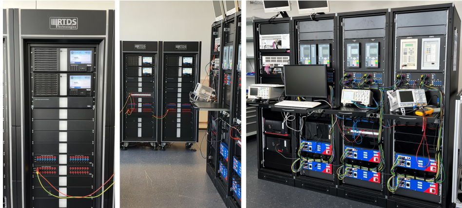
(a) Real setup consisting of an RTDS system (left) and protective devices as well as voltage and current amplifiers (right).
