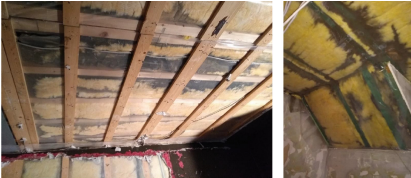
Fig. 7. Left: Ceiling over the fire source: Heavy sooting especially around the panel joints and cracks; Right: Sooting of the insulation panels in the roof, although the actual fire happened only on the ground floor.
