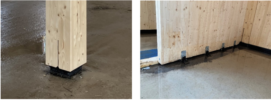
Fig. 7 Glulam column (left) and CLT wall (right) elevated above concrete slab on galvanized and painted steel bases
