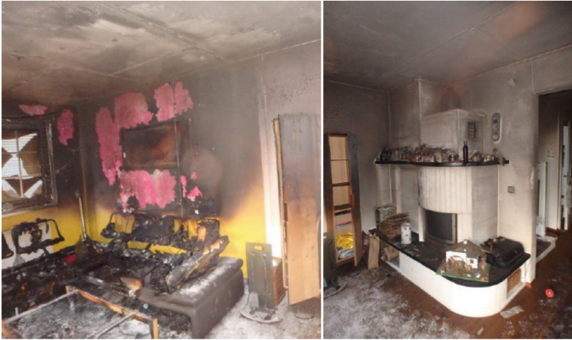
Fig. 6. Room after smoldering fire, with heavy sooting also in adjacent rooms
