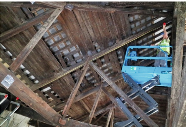
Fig. 6. ToF measurements on the lower edge of a rafter; start and end probes marked in red and yellow measuring tape covering a distance of almost 6 m.
