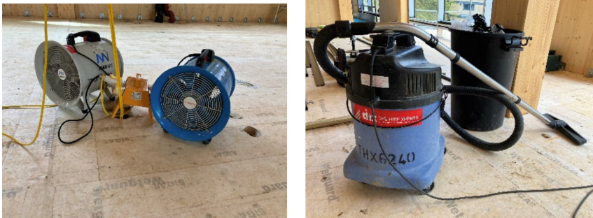
Fig. 9 Left – Fans used to promote air movement and passive drying in enclosed building. Right – Wet-vac for active water removal.
