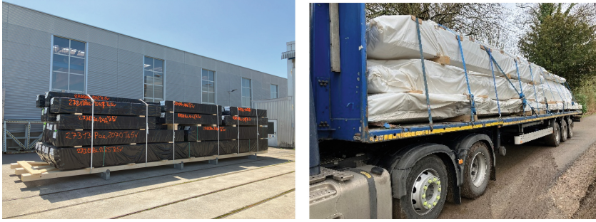
Fig. 4 Left – pre-wrapped erection-lot of glulam beams on bespoke transport skid. Right – pre-wrapped erection-lot of CLT panels as delivered to site.
