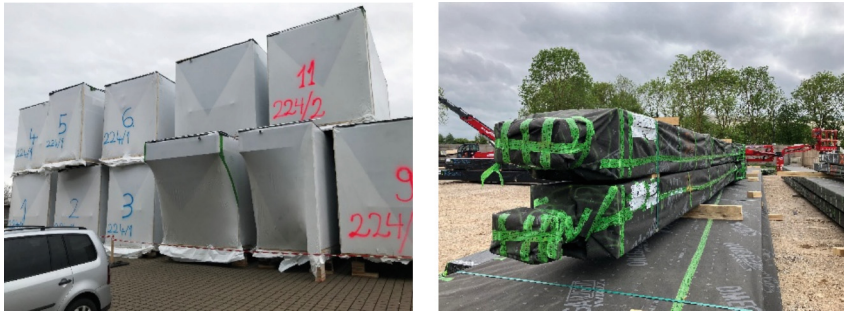
Fig. 5 Left – pre-wrapped erection-lots of timber elements stored on site, elevated and ventilated. Right – Pre-wrapped glulam beams stored on site, elevated and ventilated.
