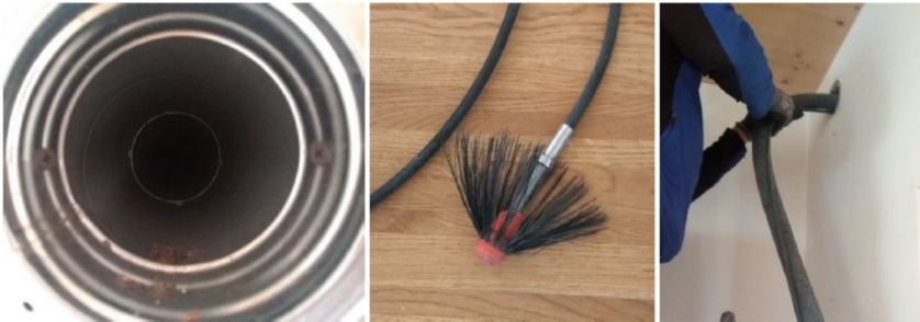
Fig. 10. Left: Soot inside air ventilation pipes; middle: Special tube cleaning brush; right: a powerful vacuum is needed
