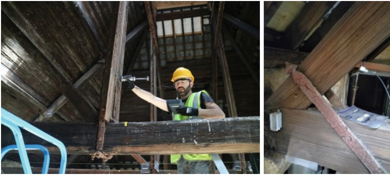
Fig. 5. Measurements of moisture content on a queen post (left) and detail of a sensor near a connection (right)
