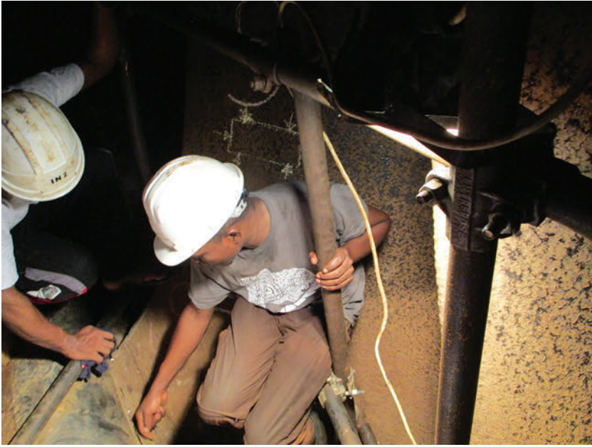
Figure 3.3. Mechanical engineers working in the Francis turbine. Photo by Barbara Carbon.
