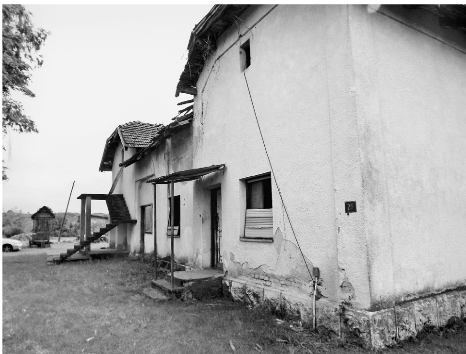
Fig. 1 Building near Donja Bišnja, Derventa, Bosnia and Hercegovina. 19 May 2016. Photograph by Kim Burton.
