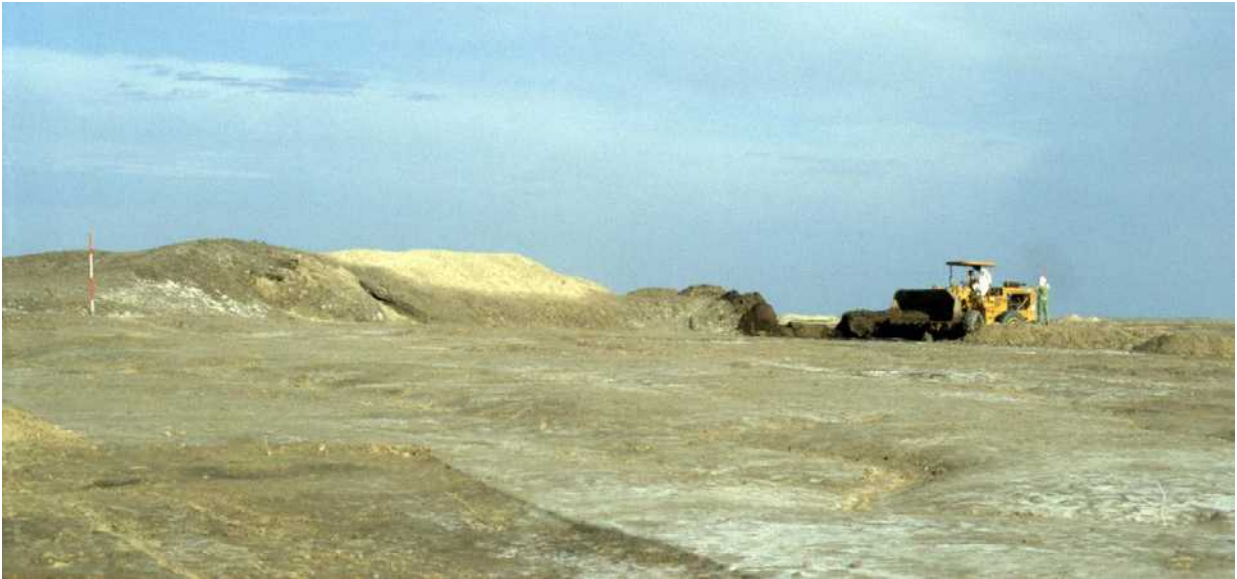
Figure 5.9. Moving the 1965 spoil heap from over the South-East Complex (view from SE in 1989).
